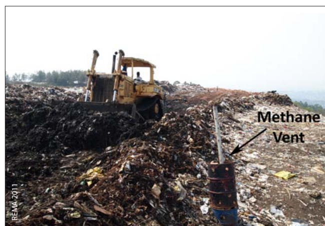
A bulldozer compacting trash at Nyanza near a vent installed to release methane
